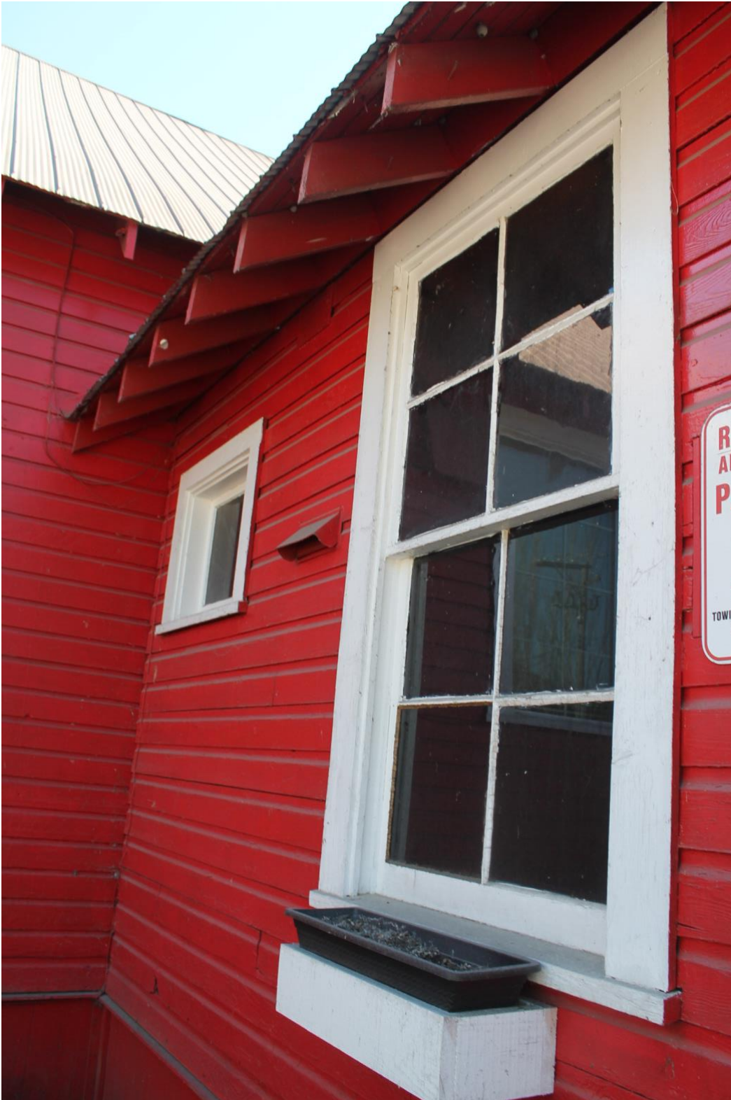
Example of wood frame and sash windows, north-facing (kitchen extension), and drop siding covering most of the building
