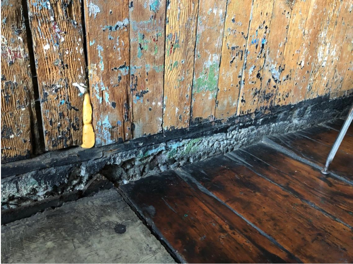
Original floor and wall components of the pass-through including rough wood wall, concrete foundation and heavy timber flooring.
