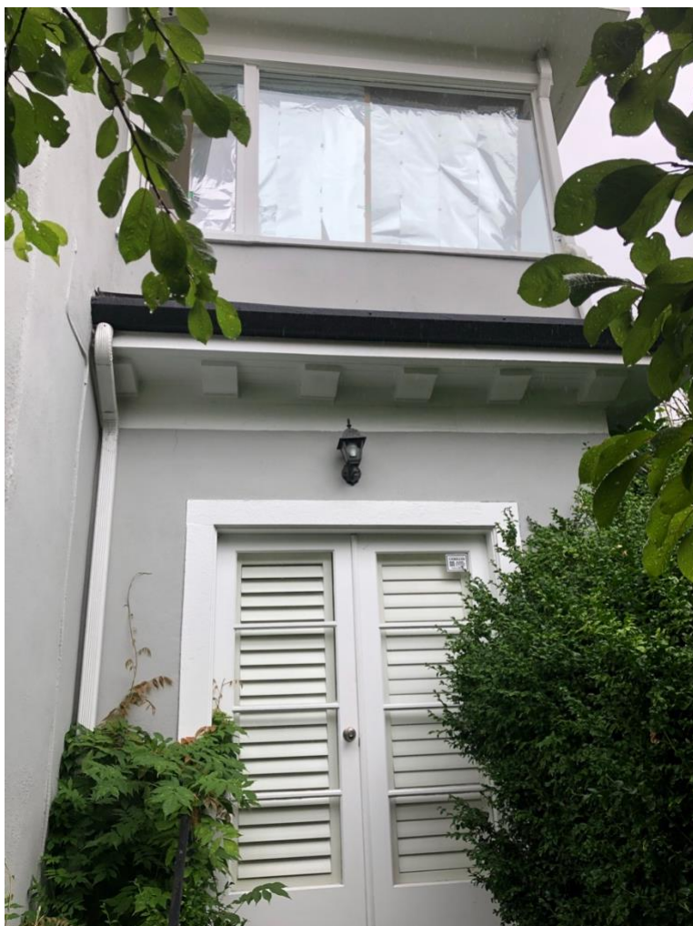
Figure 26: Paired doors accessing the library at the north end of the east side (front)
